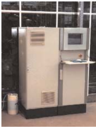
Monitoring and Control Panel
