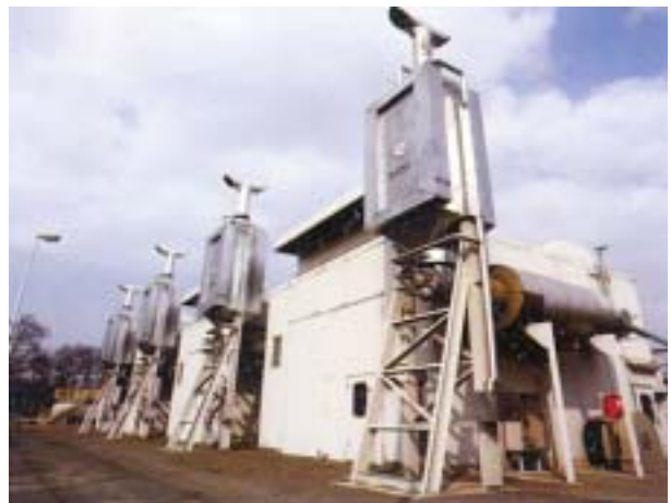
SCR/Oxidation catalyst systems to reduce \text{NO}_x/\text{CO}/\text{CH}_x from engines at a compressor station
