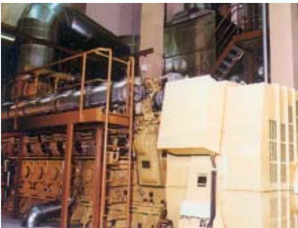
SCR catalyst system to reduce \text{NO}_x from a 7MW el Diesel engine at a cogen site
