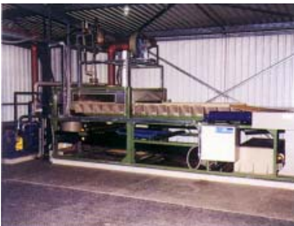
Vacuum belt filter for gypsum recovery
