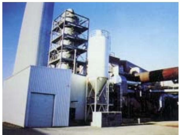
DESO x scrubber with absorbent silo and machine hall for pumps and vacuum belt filter
