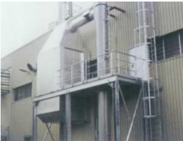
SCR/Oxidation catalyst to reduce \text{NO}_x , CO, \text{CH}_x , dioxins and furans
