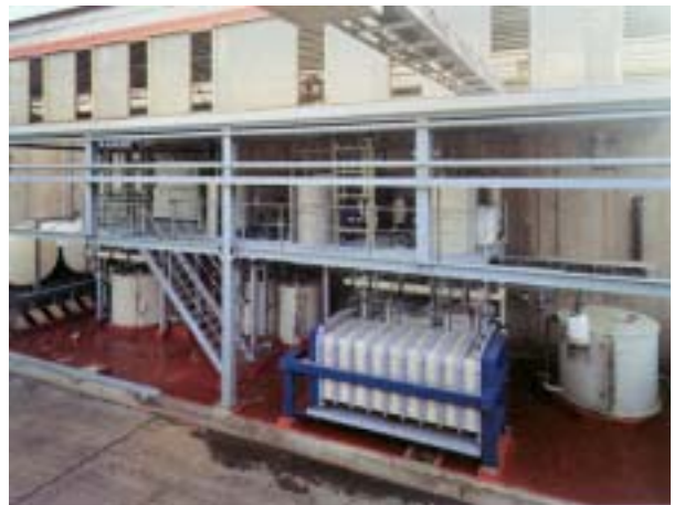
Mixed acid regeneration system
