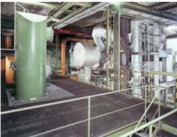
Thermal combustion chamber, heat exchanger, particulate filter and wet scrubber downstream of a special waste incinerator
